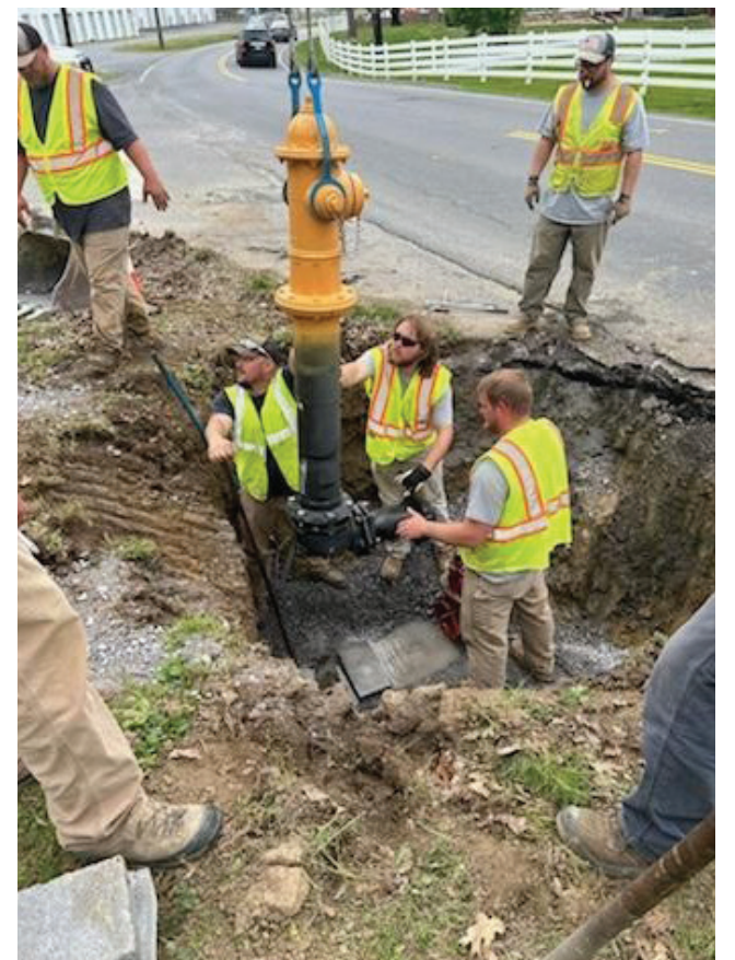
A Sevierville public works crew works to replace an aging fire hydrant.
