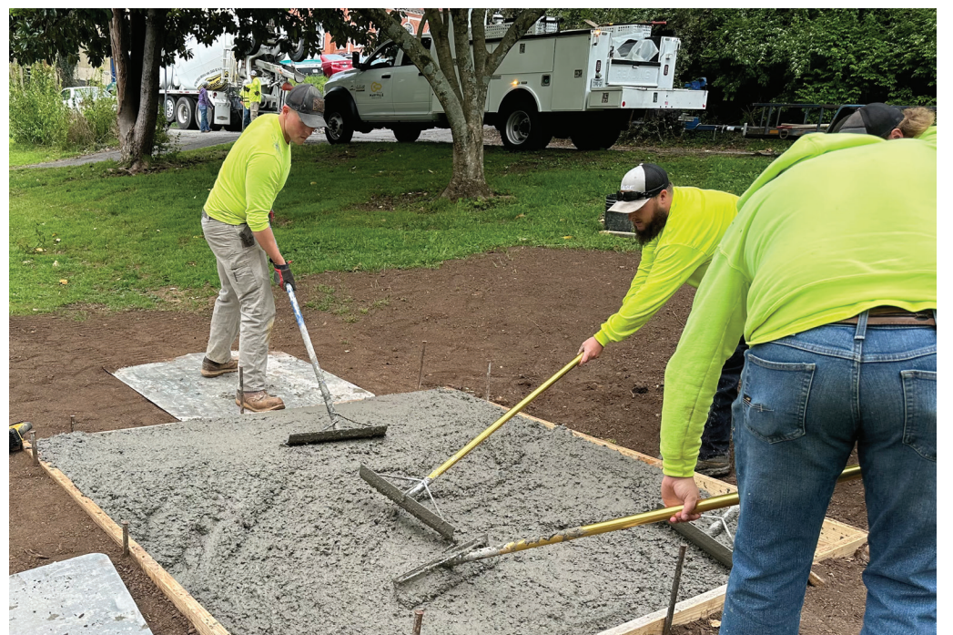
Maryville's construction crew pours concrete pads in a city park. Their work is vital for upgrades and improvements to the city's parks and recreation offerings.
