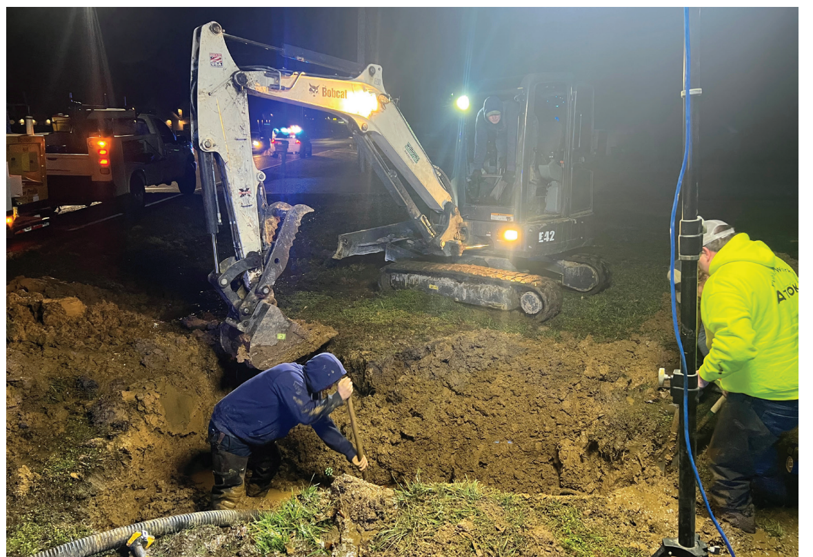
The Atoka public works team works to prepare a water line that broke during cold temperatures last January.
