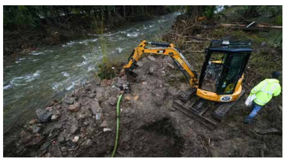
Crews with the South Elizabethton Utility District work to repair a water pipe damaged in flooding.
