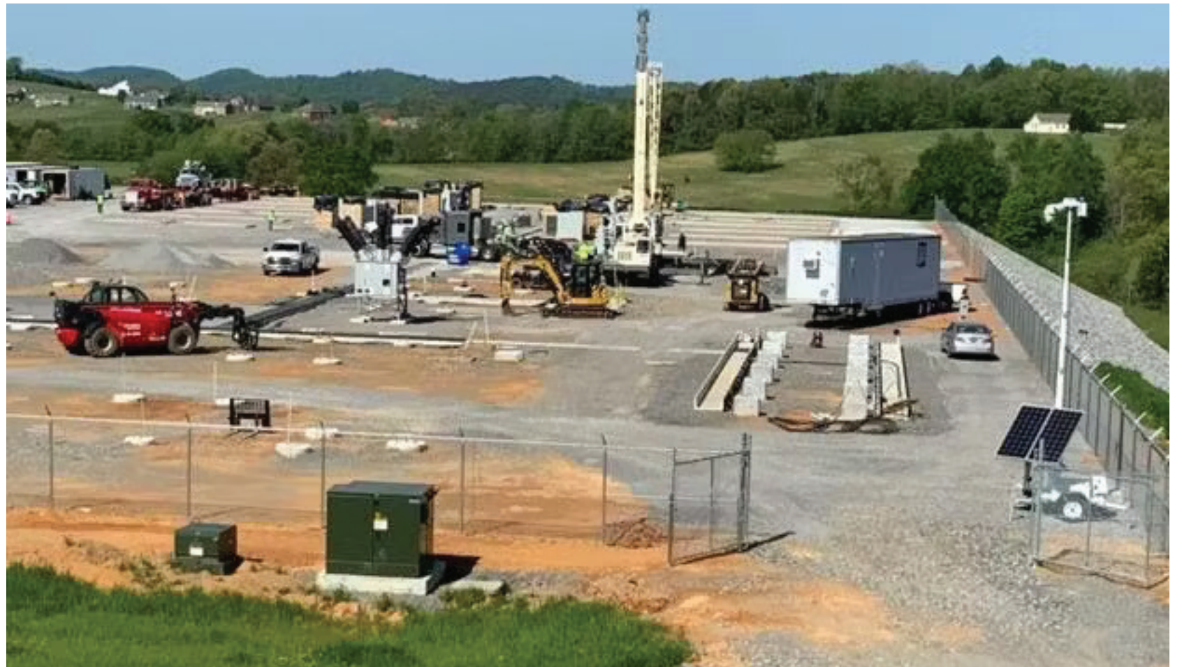
Construction is underway at TVA's first grid-scale, battery energy storage system in Vonore. When complete, the Vonore Battery Energy Storage System (BESS) will use lithium-ion batteries, the same technology used in most electric vehicles, to store 40 megawatt-hours of energy. That is enough electricity to power over 10,600 homes for three hours.
